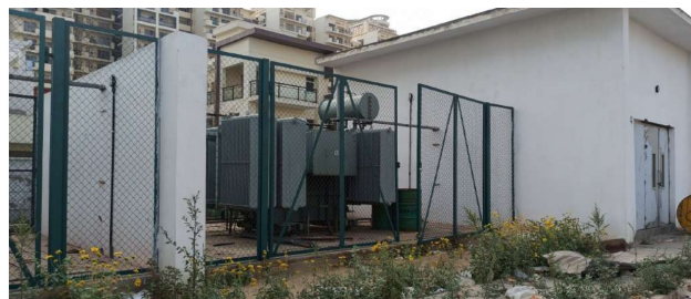
Transformer oil filtration - 5.5 MVA, 33 kV - Gurugram
