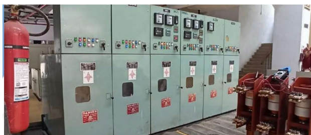
11 kV VCB maintenance & servicing - Substation, Mandi (H.P.)
